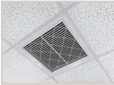
Return grill attached to filter assembly
