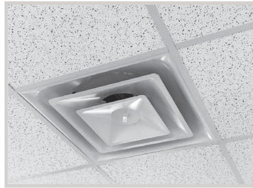
Supply diffuser(s) that connect to fan assembly
